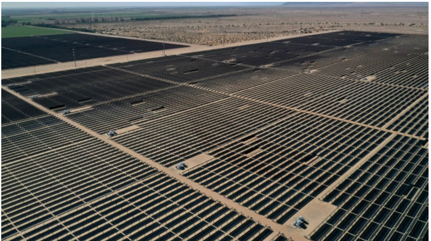
Arrays of photovoltaic solar panels are seen at the Tenaska Imperial Solar Energy Center South in this aerial photo taken over El Centro, California, U.S., May 29, 2020. Picture taken with a drone.
